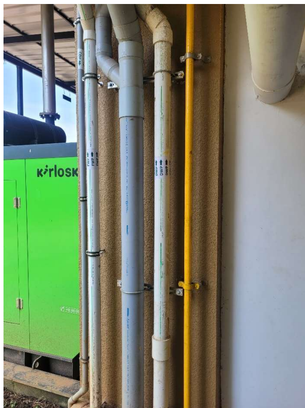
Dual Plumbing line
