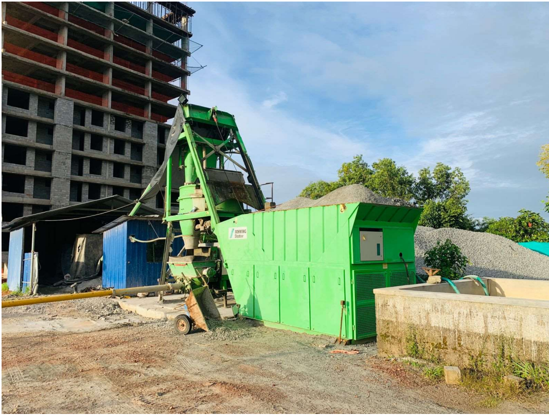
Concrete Mixing plant Annexure No.9.
